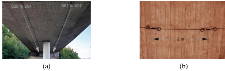
Figure 3. Overview of the bridge and the monitoring system: (a) Sensor distribution; (b) An LGFBG sensor with a 2.05 m gauge.
